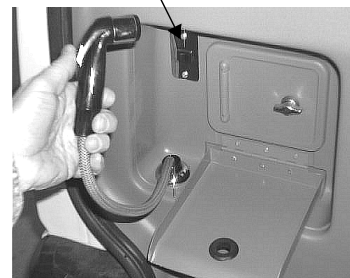
Water Pump Switch
