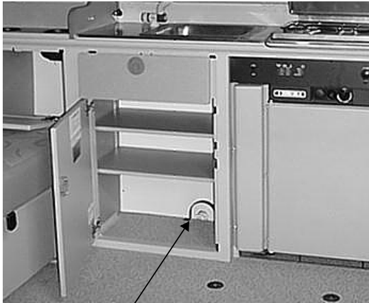
Water Line Drain Valve
